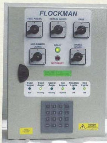
Flockman controller enclosure
